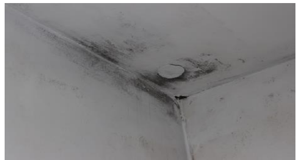
Damp on walls, ceiling and windows in all three Bedrooms
