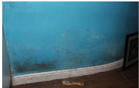
Damp and black mould in evidence in kitchen (rear ground floor)
